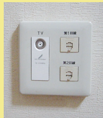
Modular jack (in apartments where two lines can be used)
